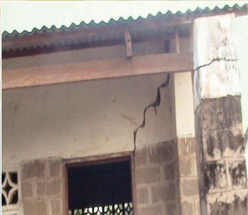
Abandoned Class block - Chikunkha Primary School, Nsanje District
